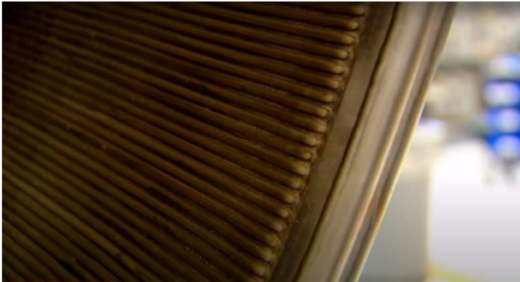
Figure 36: Cold fuel passing through tubes inside the nozzle
